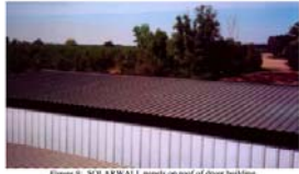
Figure 9. SOLARWALL panels on roof of dryer building
