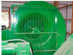
Burner after fan
