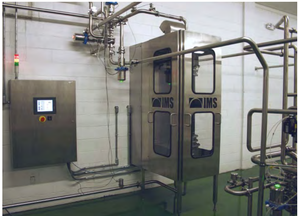
Control panel and two-stage microwave heater at Yamco production facility.
