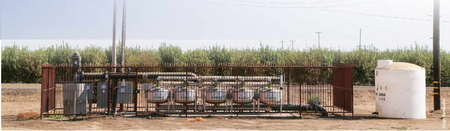
A groundwater pumping system in Merced County.
