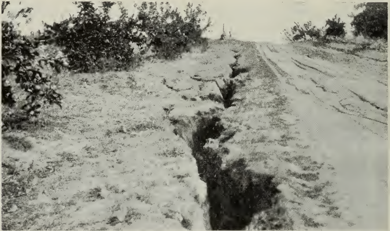
Fig. 29.—The orange grove on the left is protected, by means of terraces, against erosion, but a satisfactory terrace outlet has not been provided, with the result that a shallow drain along the driveway has become a gully.
