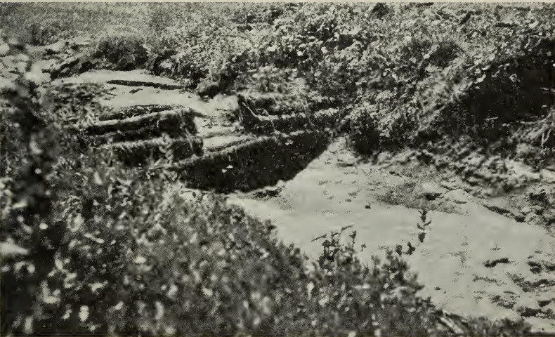
Fig. 33.—A soil-saving dam of small poles firmly bound together with wire cable. Note the notch left for the passage of water so as to prevent its cutting around the ends of the dam. Photograph taken July 5, 1929. (See fig. 34.)
