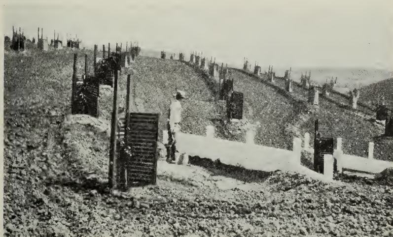
Fig. 30.—Well-constructed wooden check dam with tile underdrain and riser being used to prevent a gully from forming at the end of terrace runs. Steep hillsides can be planted safely in this way.
