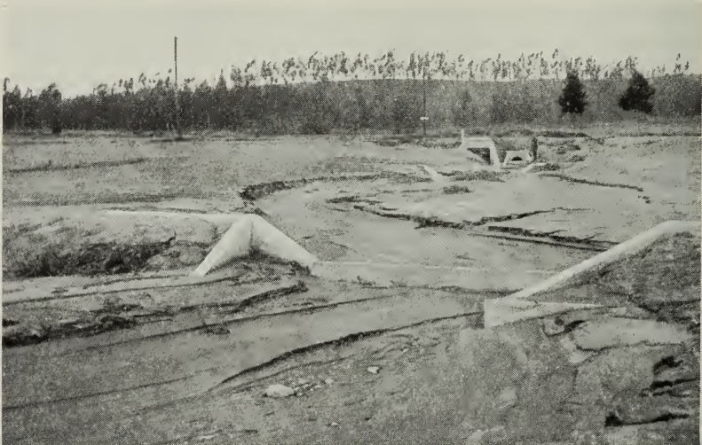
Fig. 35.—These concrete soil-saving dams in Ventura County will prevent this gully from becoming deeper, and although the channel may continue to carry storm water there will be no further loss of land.
