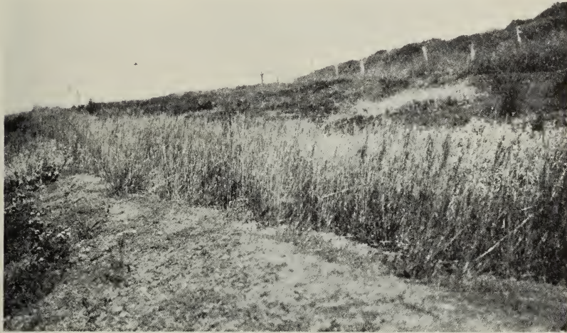
Fig. 36.—A gully in the early stages of formation was prevented from getting beyond control by the construction of rock check dams and seeding the sides to native grasses. (Photograph courtesy A. W. Sampson.)
