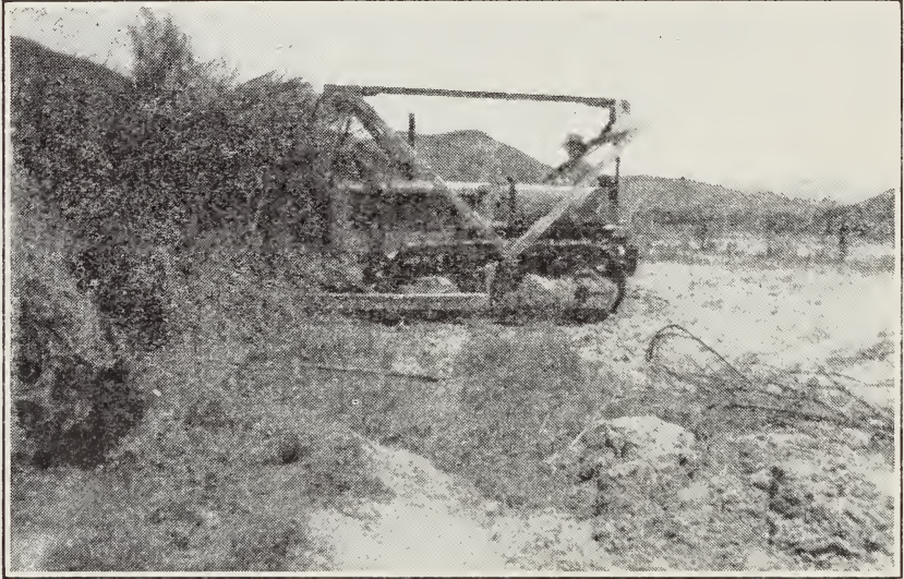
Fig. 14.—Use of a bulldozer for clearing brush lands. (Compare with figures 10 and 11.) The uprooted brush is piled for burning later; small piles may be left as shelter for quail. (Photograph by Cliff Topham.)
