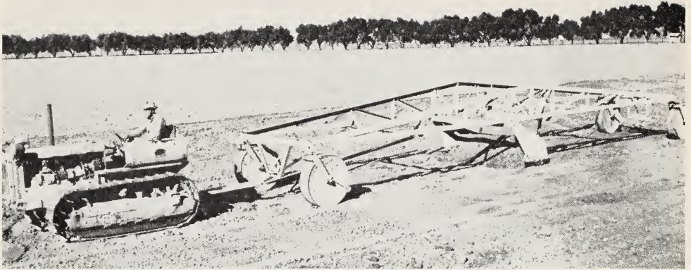
Fig. 5.—Land planing is done after field has been rough-leveled, to insure that minor irregularities are eliminated. Careful leveling permits efficient use of irrigation water.
