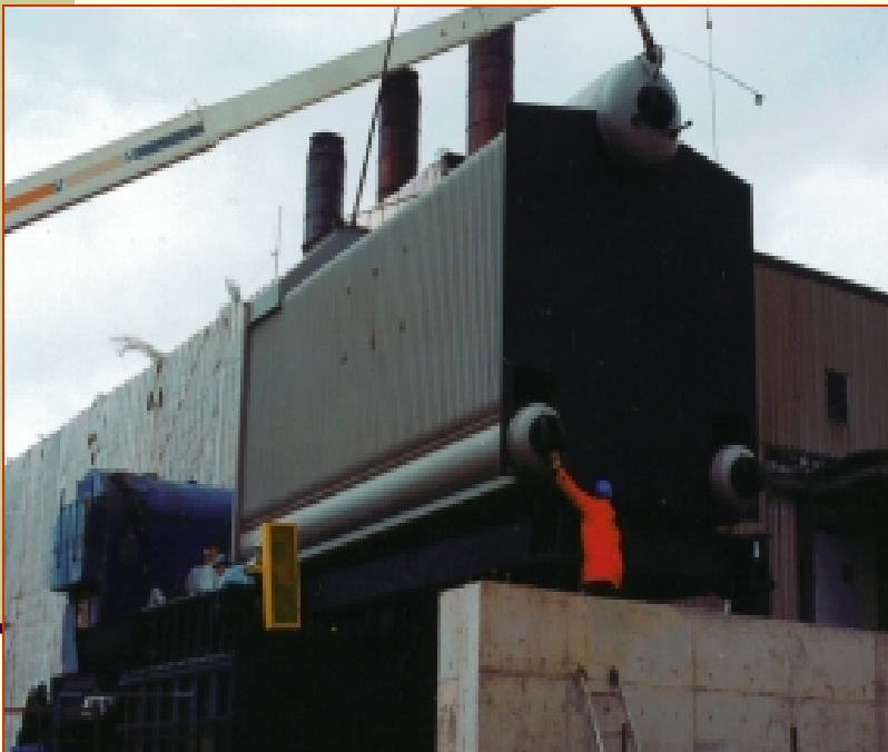
Itasca Power 20 MW Plant Prince Edward Island, Nova Scotia
