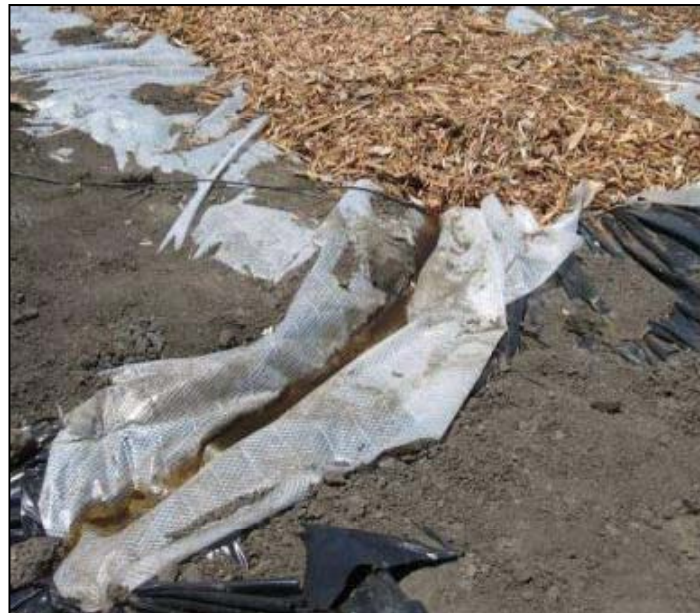
DBR outlet drains into surface ditch after approximately 2 days of residence time
