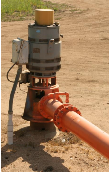
Well water (2 to 70 ppm Nitrate-N)
