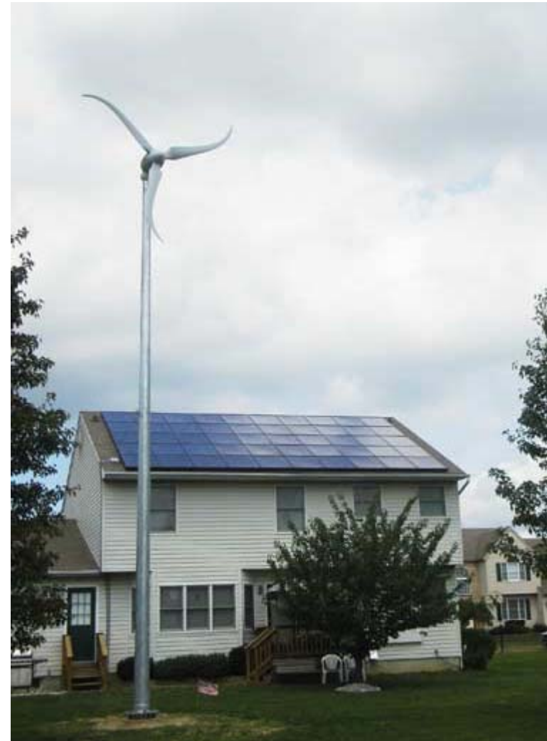
Source: Southwest Windpower
