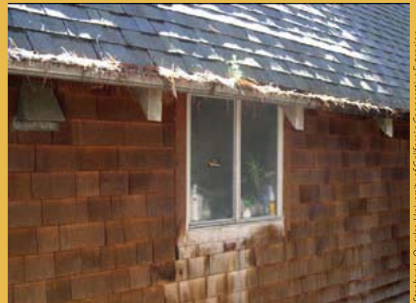
Accumulated fuel in rain gutter.
