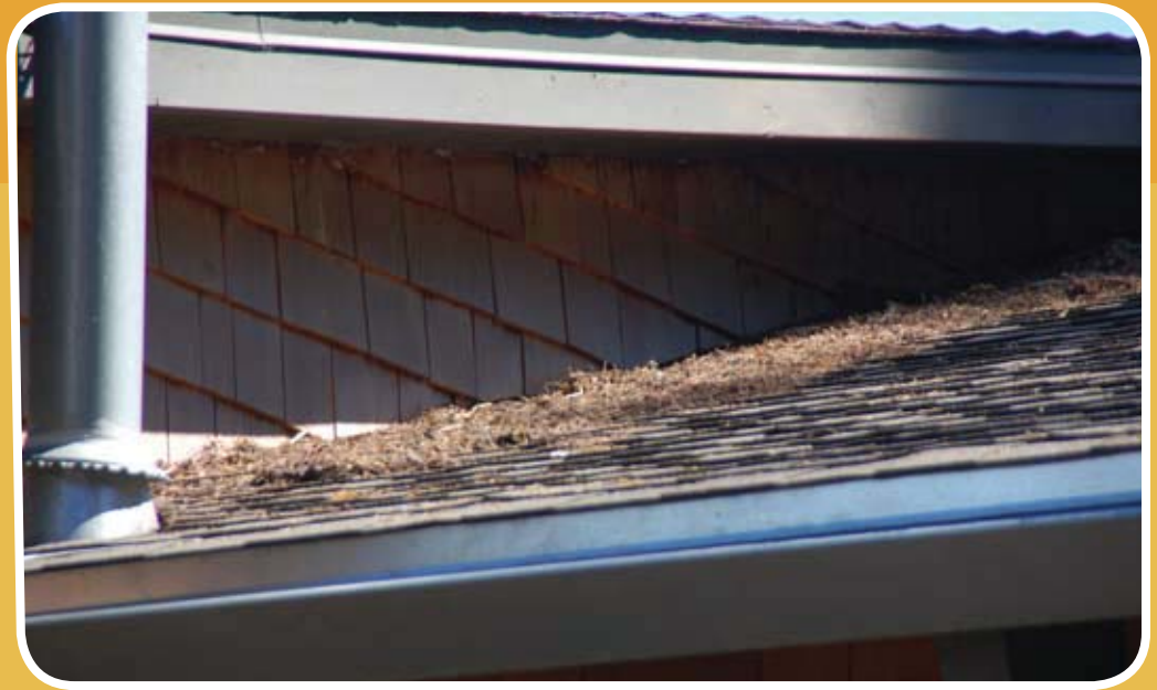
Accumulated pine needles on this complex roof could allow embers to ignite roofing materials.
