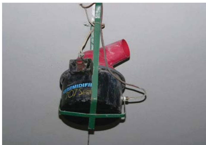
A storage room humidification unit
