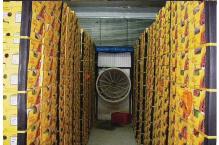
Forced-air cooling tunnels
