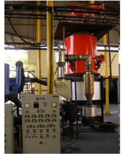
Ankur derivative downdraft gasifier, gas scrubbing/filtering, recip. engine-generator (~500 kW)
