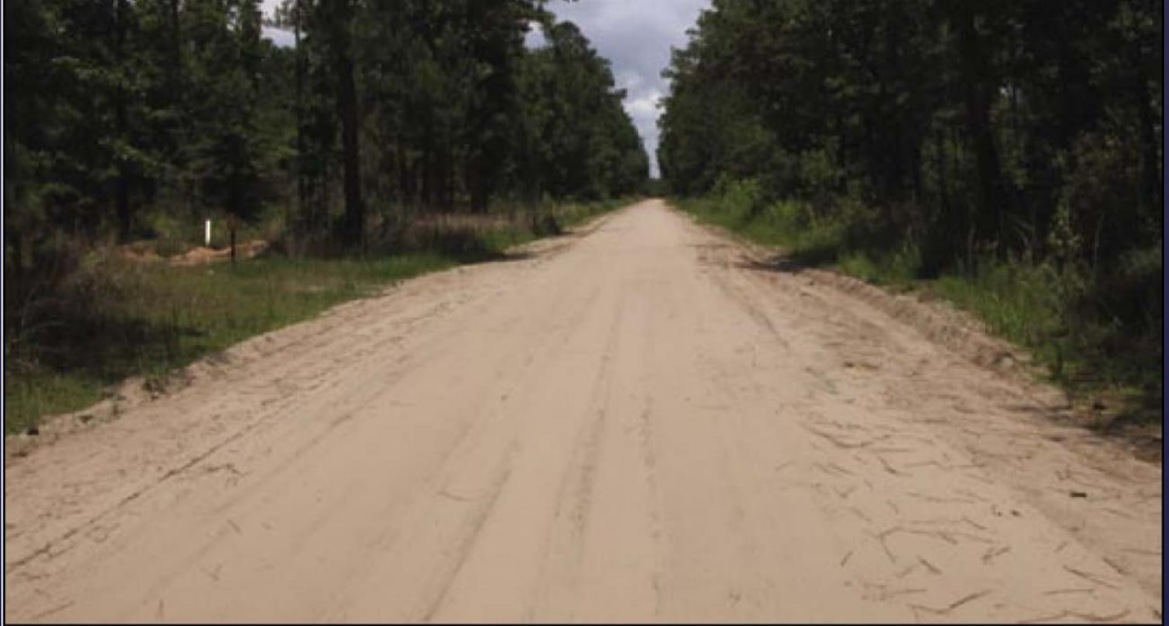
Figure 18—Maintenance level 3 road with double lanes and native road surface with shoulders.
