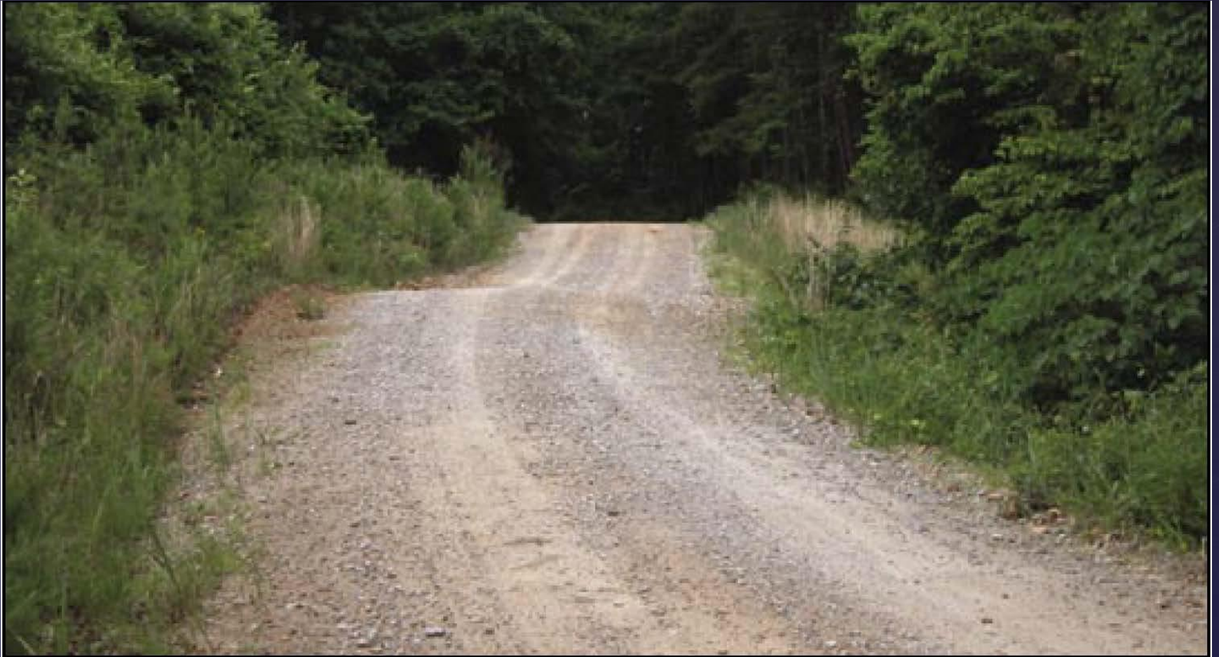
Figure 16—Maintenance level 3 road with single lane, gravel surface, no shoulders, and a cross drain dip.
