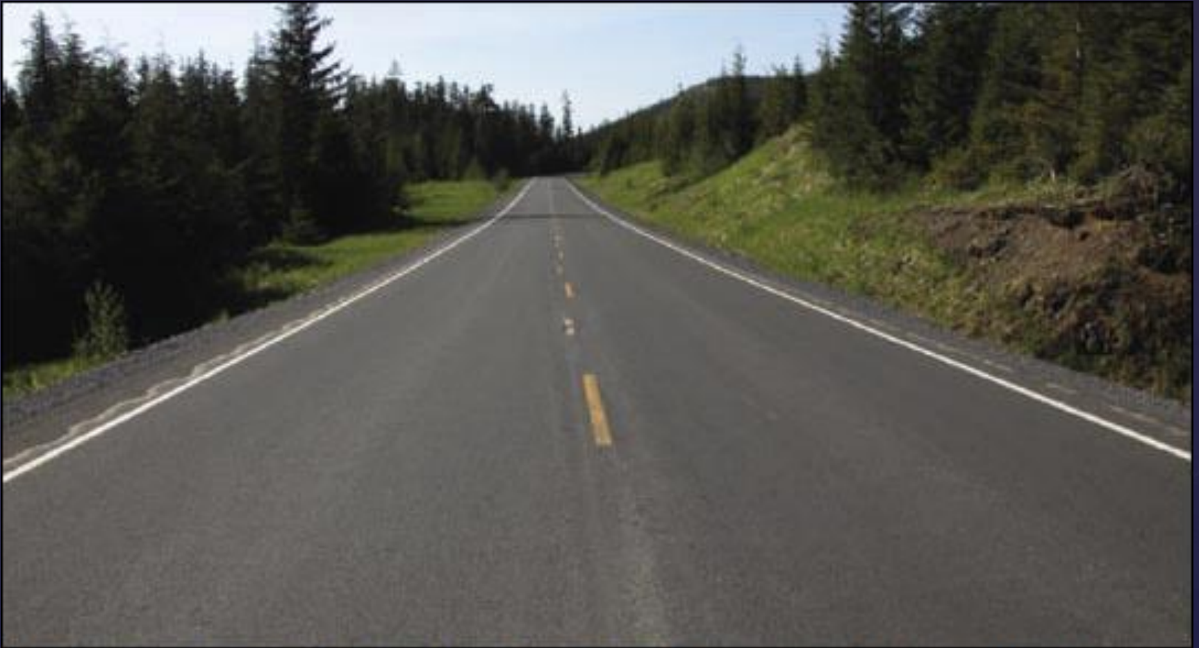
Figure 1—Maintenance level 5 road with double lanes, hot-mix asphalt surface, and asphalt- and rock-stabilized shoulders.
