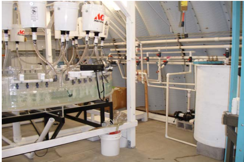
Figure 21. Water preparation and distribution systems.
