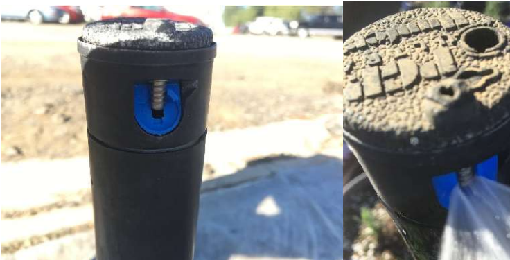
Figure 4. Different nozzles installed (see number 4 and 6 printed on the nozzle).
