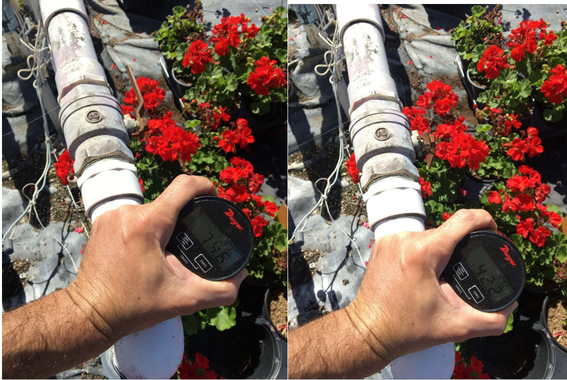
Figure 3. Example of “throttling”. The pressure was 74 psi and by partially closing a valve we reduced it to 42 psi. The same result can be achieved with a pressure regulator.
