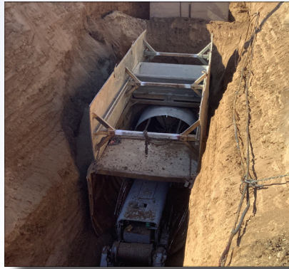
Left: Cast in place concrete pipe machine
