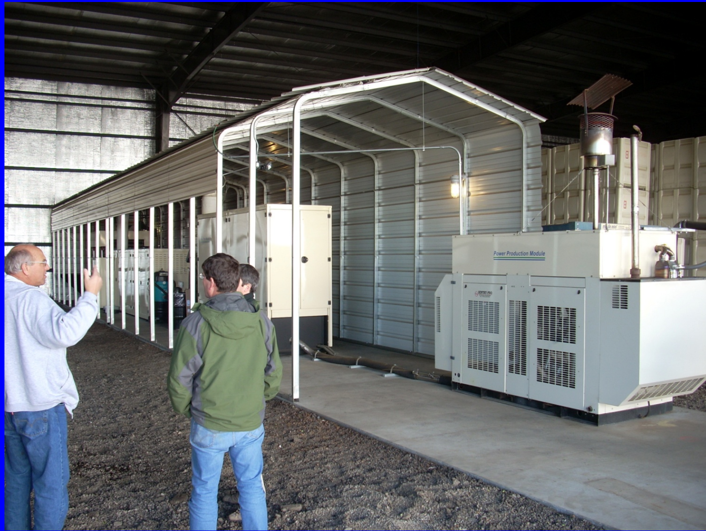
Biomass Gasification Unit coupled to an Internal Combustion Engine and Generator - 500 Kw
