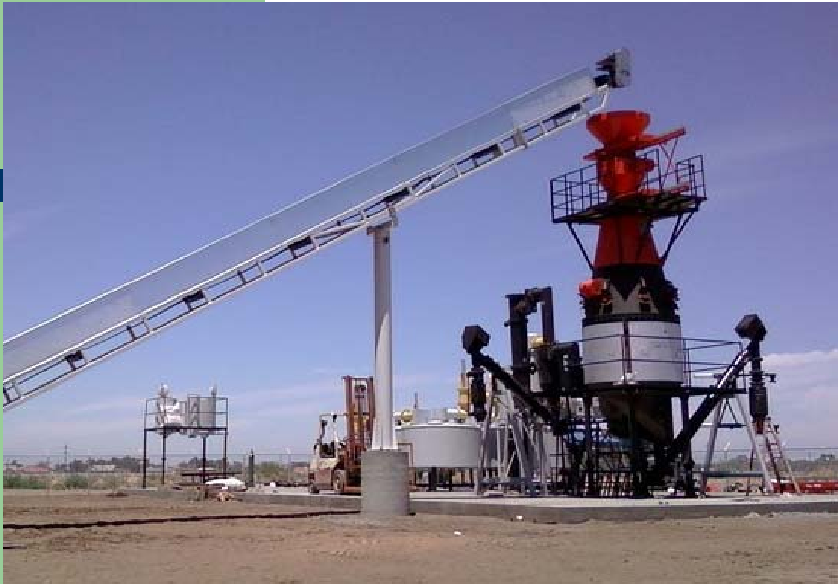
Phoenix Technologies Biomass 500 kWh Gasification Unit at Madera
