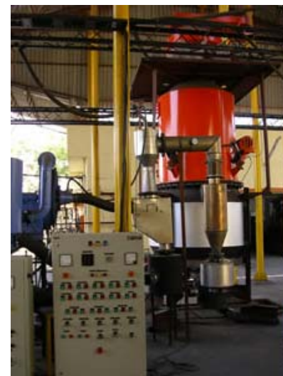
Ankur derivative downdraft gasifier, gas scrubbing/filtering, recip. engine-generator (~500 kW)
