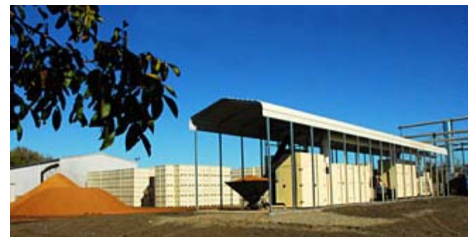
Downdraft gasifier, gas filtering, automotive V-8 engine-generator (~50 kW)
