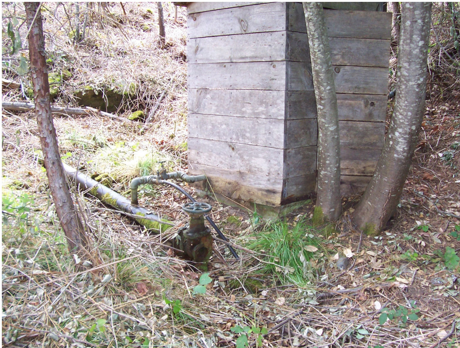
Outlet pipe and valve at downstream toe of dam. (8/16/05).
