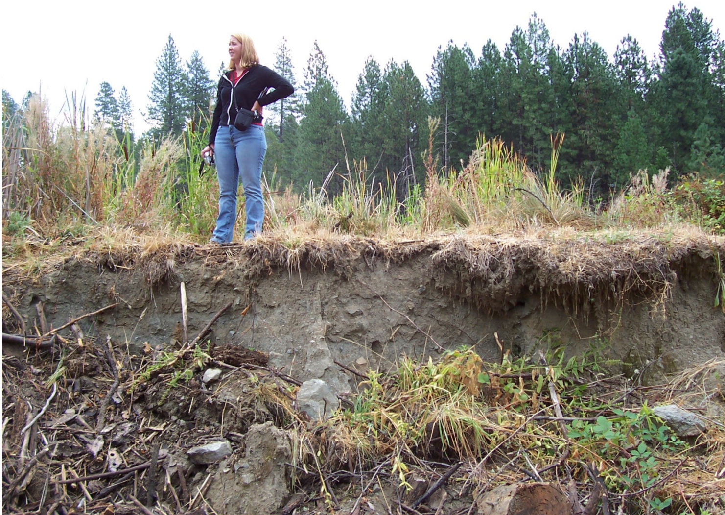
View of vertical face of headcut at top of embankment (8/16/05).
