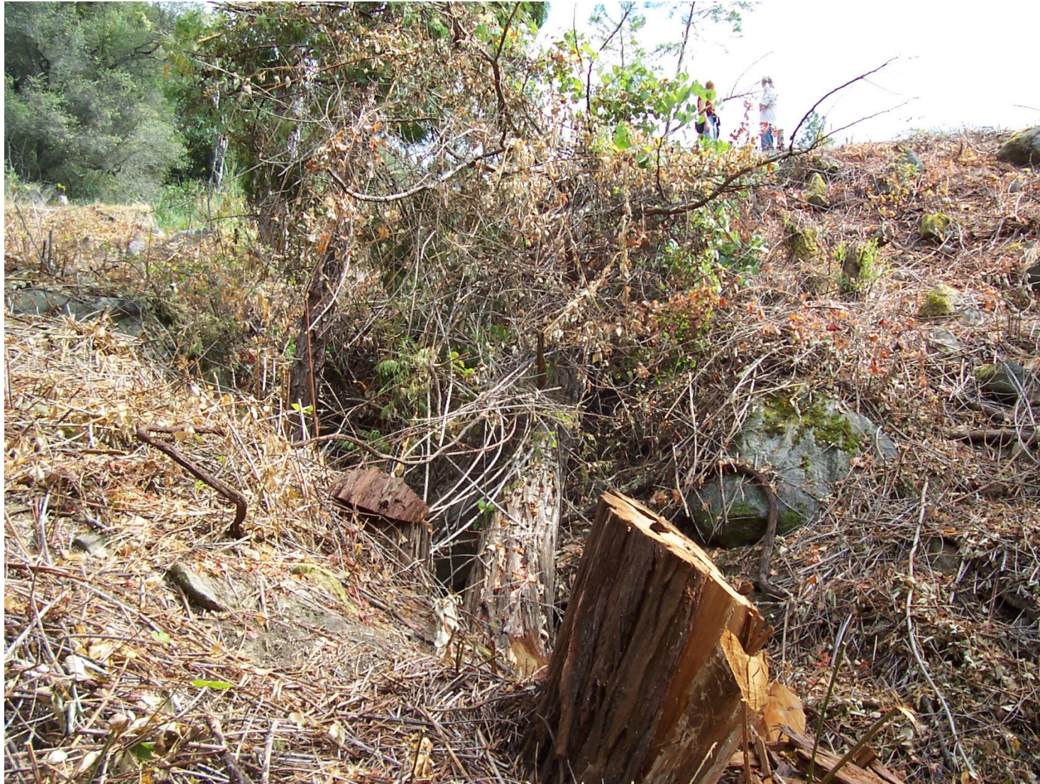
Vegetation to be cleared from lower portion of eroded embankment (8/16/05).
