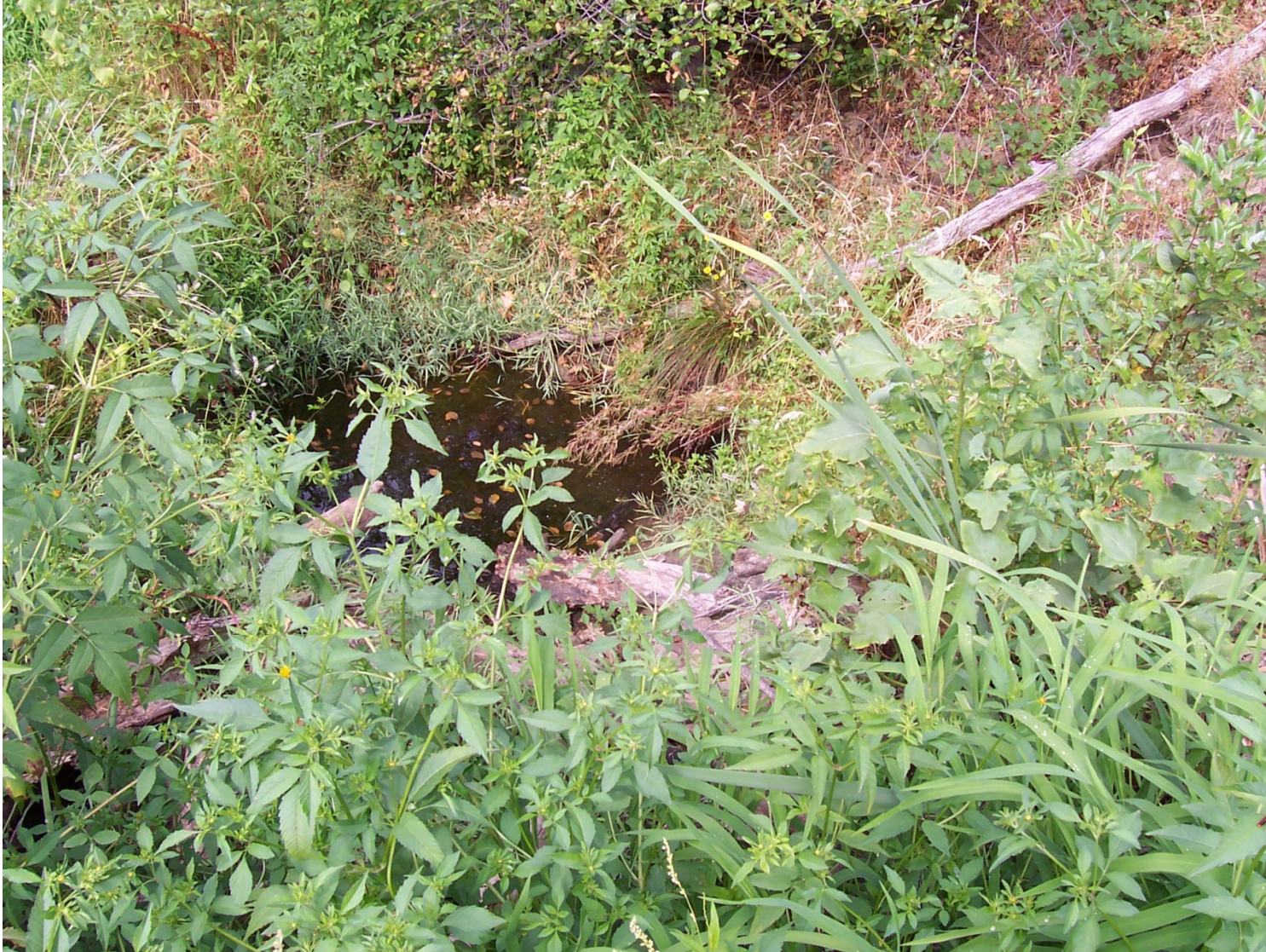
Standing water in emergency spillway exit channel. Flow from right to left. (8/16/05).
