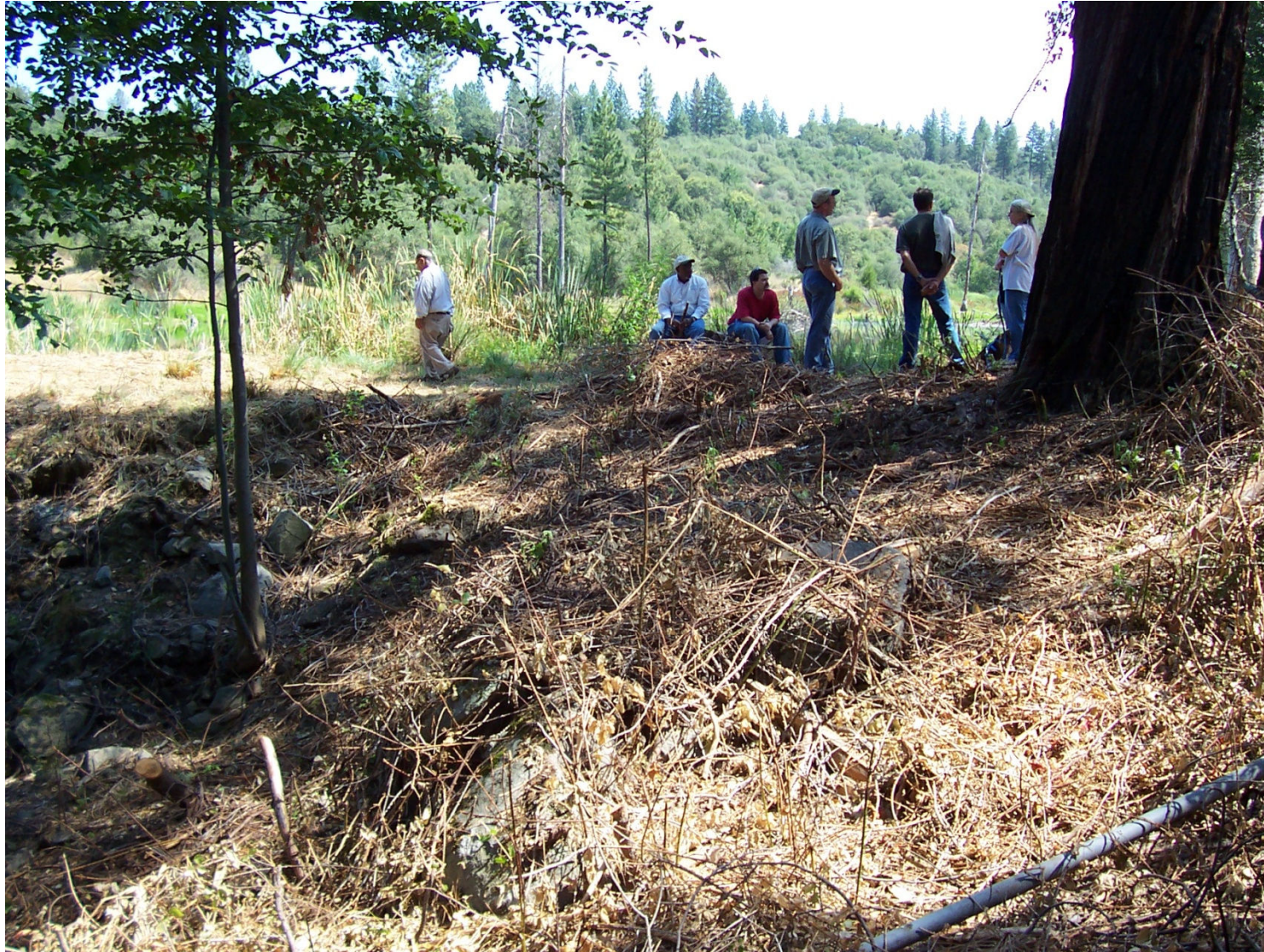
View of minor erosion to downstream face of embankment near south abutment past small tree. (8/16/05).
