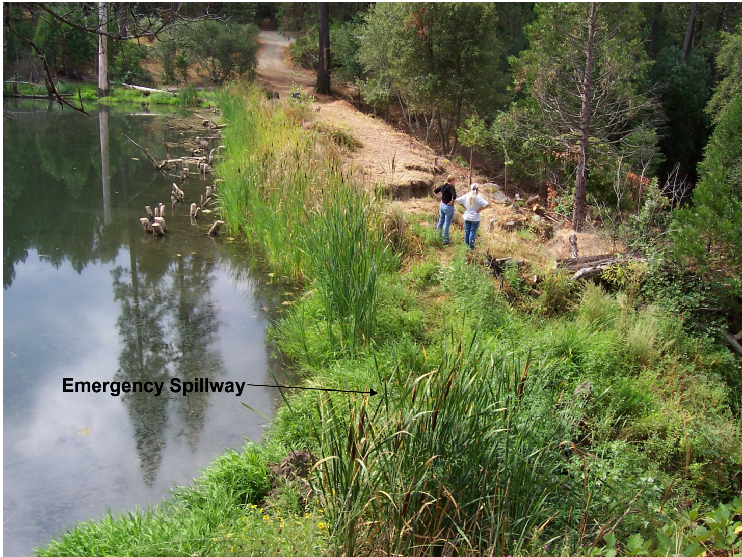
View of erosion to top of embankment, trees on embankment and vegetation in emergency spillway (8/16/05).
