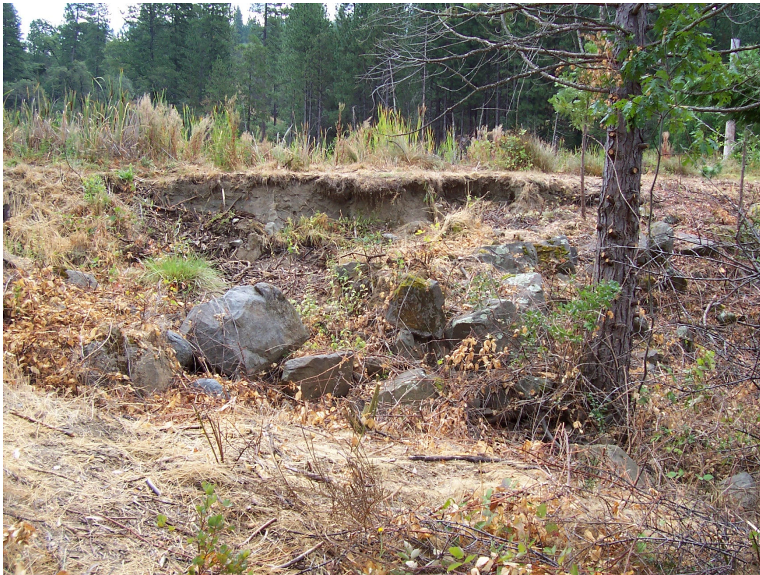
View of erosion to downstream face of dam (8/16/05).
