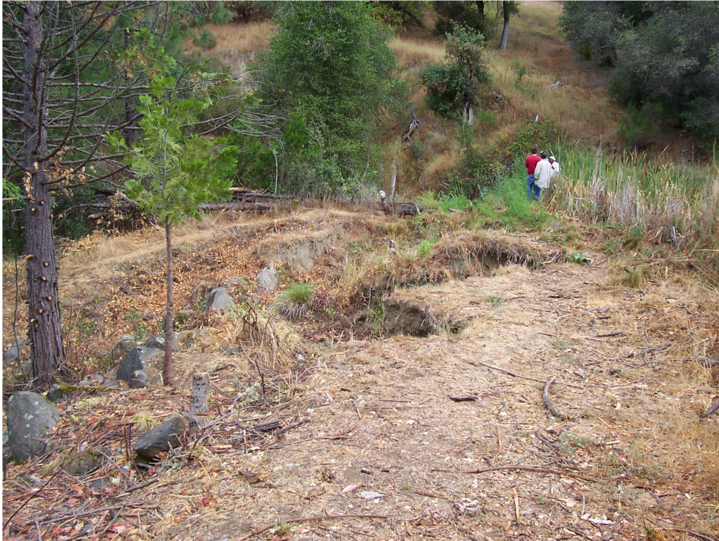
Top of embankment looking north at erosion to top of embankment (8/16/05).
