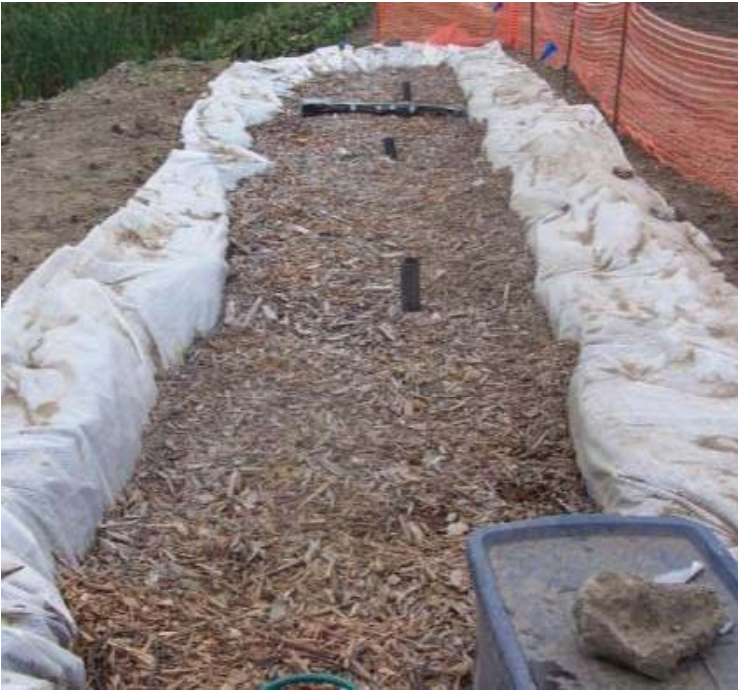
Denitrification Bioreactor 1 (DBR 1) 930 cubic feet
