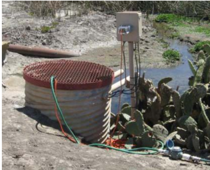
Continuous pumping into DBR from tile drain sump
