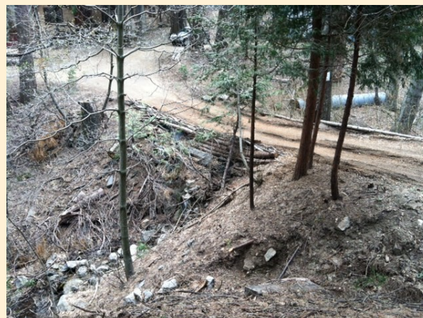
Forest road in need of crossing and culvert improvement
