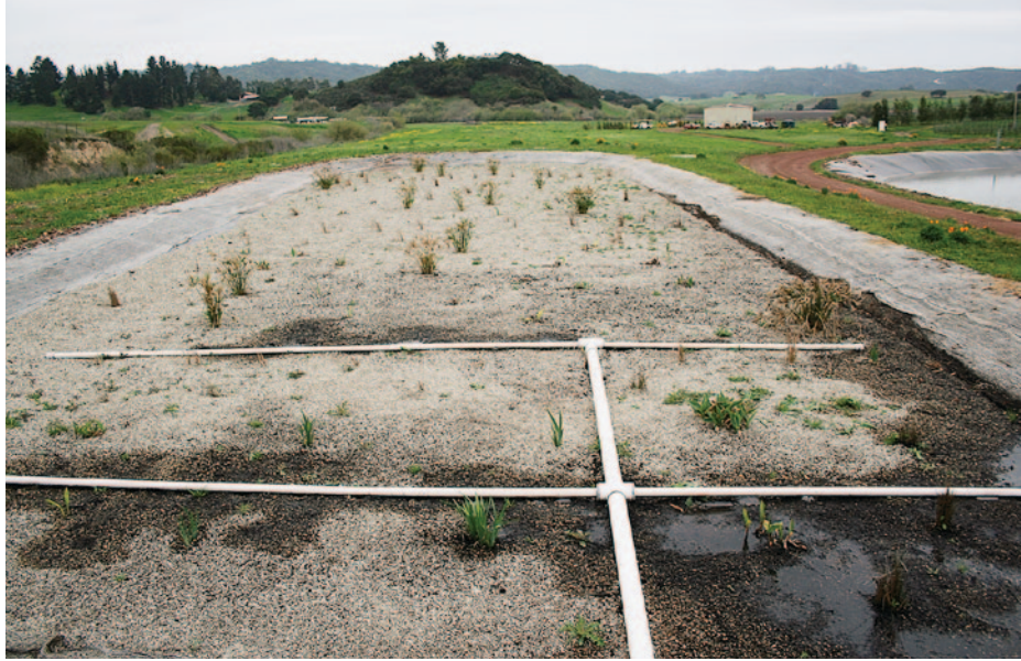
Piping disperses process wastewater across the width of a constructed wetland at a Paso Robles winery. Samples were taken at the outflow (not shown) and the far end of the wetland, which was designed to handle wastewater generated by producing 14,000 cases of wine.
