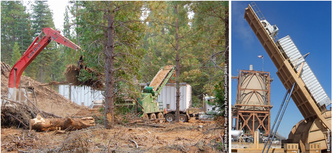
Fig. 1. At Blodgett Forest Research Station, an excavator (left) loads forest slash into a horizontal grinder. Wood chips from the grinder are then conveyed into chip vans (center) for transport to Buena Vista Biomass Power plant (right).
