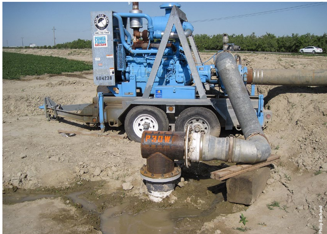
Pumps and engines were connected to piping to pull floodwater onto agricultural fields from the diversion canal on the James Bypass.
