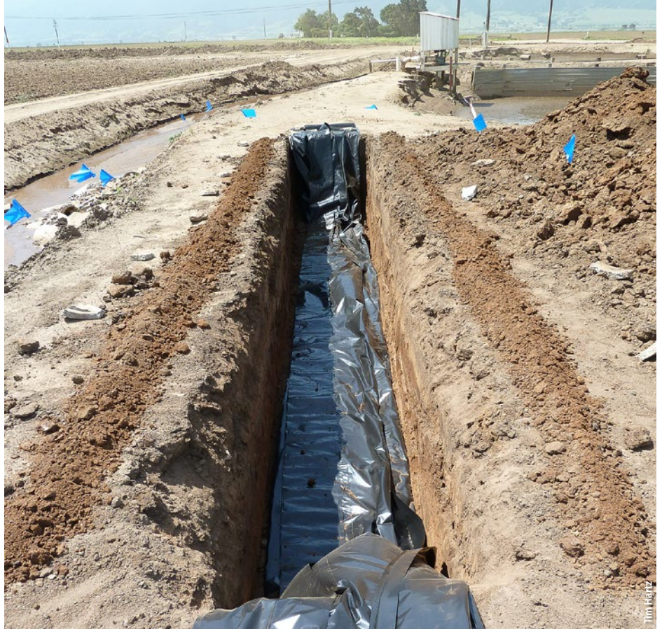
The denitrification bioreactor was dug with a backhoe and fitted with a polyethylene liner.
