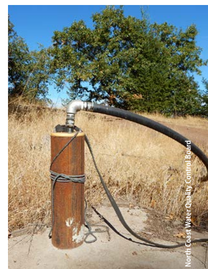
Wellhead at a permitted cannabis cultivation site.
