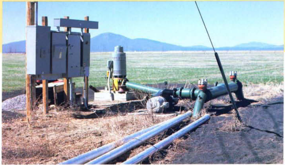
Many California farms use pumping plants to facilitate irrigation. In order to save energy, the state has initiated a program to test and improve pump efficiency.
