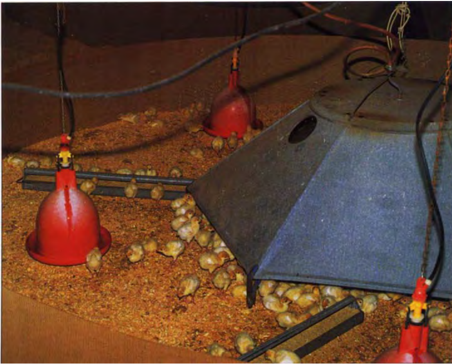
In the trials, two columns of brooder stoves were placed 6 feet from the outside wall and 8 feet from the center of the house. In this view, stoves have been raised to the ceiling. PVC pipes on the center posts hold temperature sensors.
