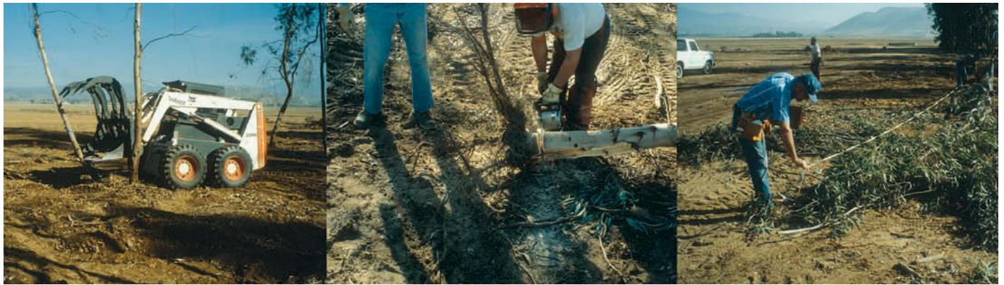
Left , record trees were pushed over and pulled up with a skid steer loader, then, center , the trunks were cut just above the root mass
