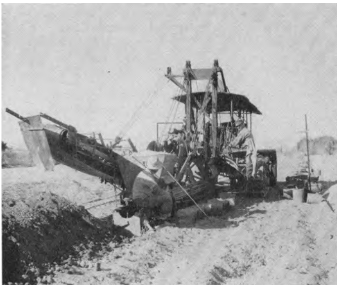
A tile laying machine used in the installation of a drainage system in the Coachella Valley.
