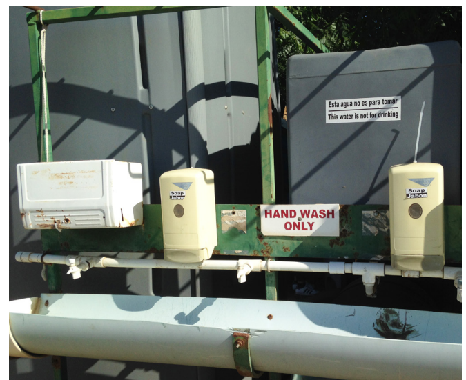
Hand Washing Station, Riverdance Farms
