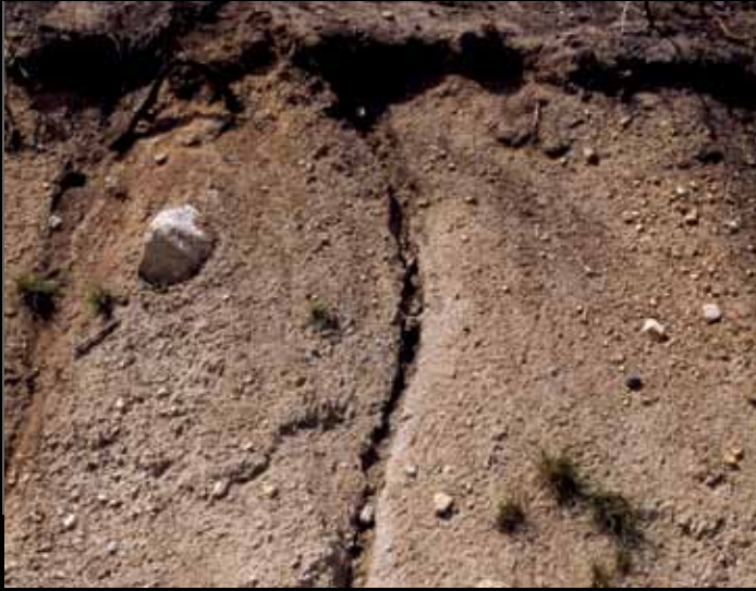
Erosion – Surface erosion.
