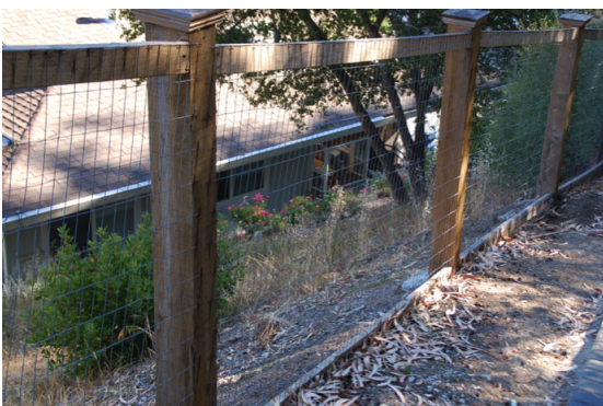
Wood frame fence with metal mesh infill. Debris accumulation at base of fence, against the wood lateral member, would make that member more vulnerable to an ember ignition, and increase the opportunity for fire to spread laterally. Source: firecenter.berkeley.edu/bwmg/attachments-1.html
