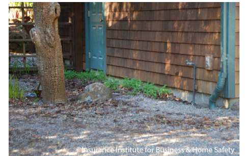
Clearance between the ground and the start of the siding should consistently be at least 6 inches.
