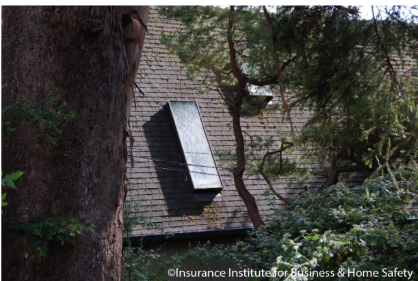
Skylight on a steep-slope roof. Radiant heat exposure from burning vegetation or building would be more of a problem with steeper sloped roofs.
