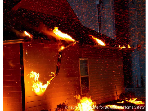
Wind-blown embers ignited debris in a gutter. Photo shows detaching vinyl gutter (left side) and attached metal gutter (right side).
