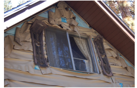
Deformed vinyl siding from a radiant heat exposure from a nearby burning home. Source: Stephen L. Quarles
