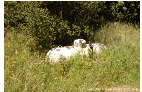
Poor defensible space near a propane tank. Ignition of this vegetation would provide a longer exposure to heat. Depending on level of fuel in the tank, an explosion would be possible under this scenario.
