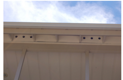
Gaps between the blocking and framing in the unvented truss bays would allow ember entry into the attic space. A sealant could be used to close gap. Source: Stephen L. Quarles
