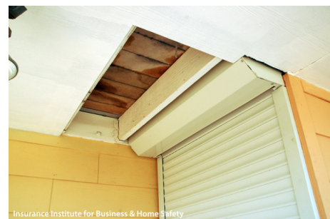
A horizontal enclosure, such as that shown here, can result in moisture-related degradation of wood and metal fasteners when deck boards are used.
