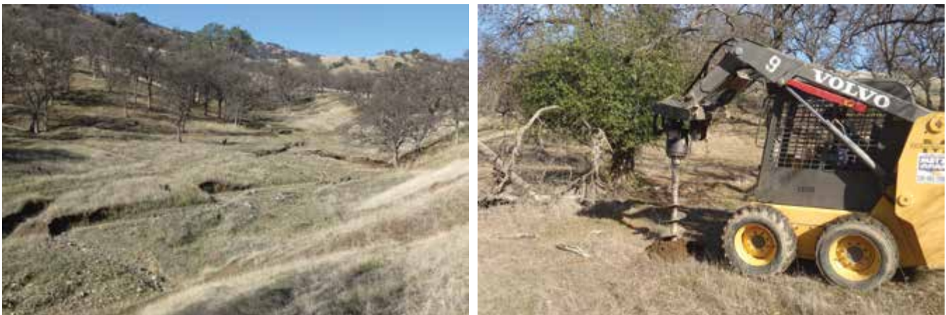
FIGURE 7. Auguring 1- to 2-ft deep holes prior to planting seedlings or acorns. The landscape view shows the slope of the terrain that permits access with the excavator/digger machinery.
