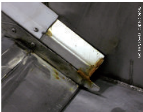
This new line has a clear design flaw, showing junction gaps and trapped crop tissue still present after cleaning. It would be considered a safe harbor site for Listeria.
