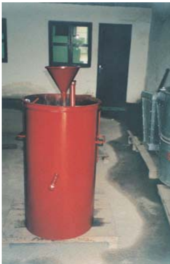
Fig. 13. Clarifier tank (O.P.C., Cameroon)
