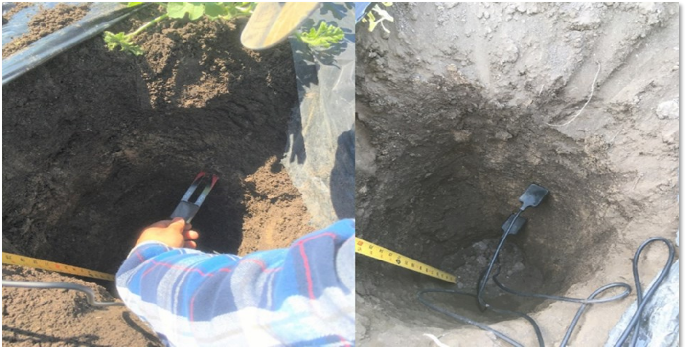
Photo 1. Installation of capacitance soil probe water sensors at a depth of 12, 18, and 24 inches in a clay soil near Stockton, CA.
