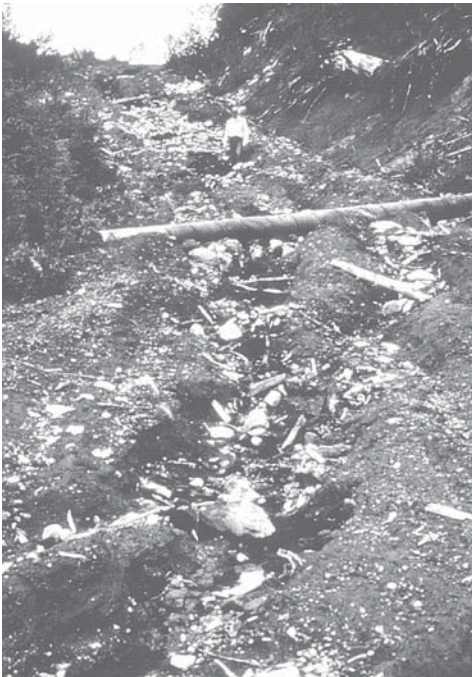
Figure 6-10. Catastrophic ditch and roadway erosion.
