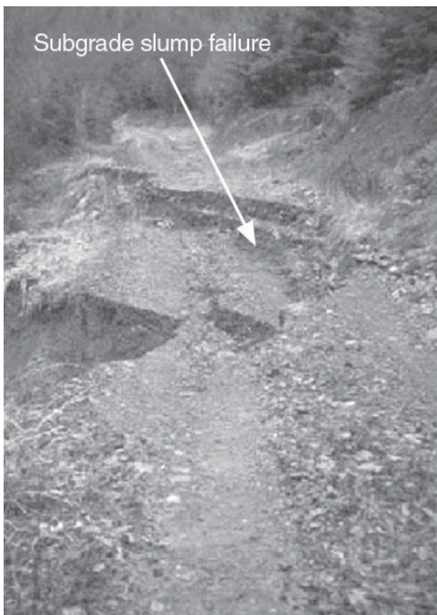
Figure 1-11. Example of a poor road location, causing a roadway slump failure.
