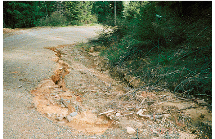
Figure 9. This ditch and road surface erosion was caused by inadequate spacing of ditch relief culverts. Photo: Susie Kocher.
