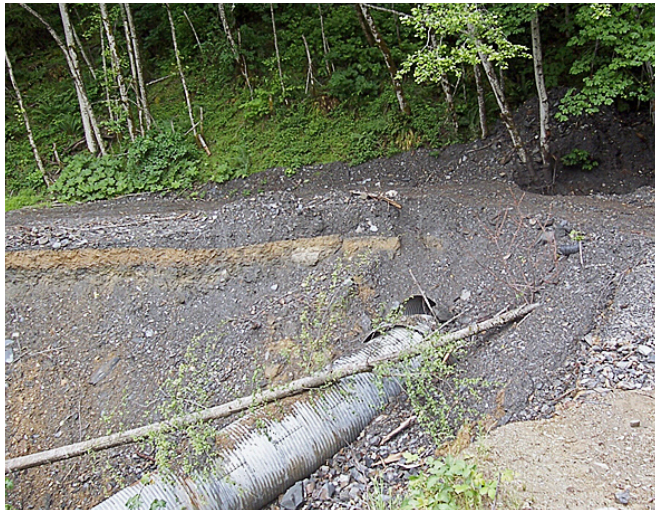
Figure 1. Culverted stream crossings may plug during storms. Diverted stream flow then crosses the road and erodes the fill slope. Photo: Richard Harris.
