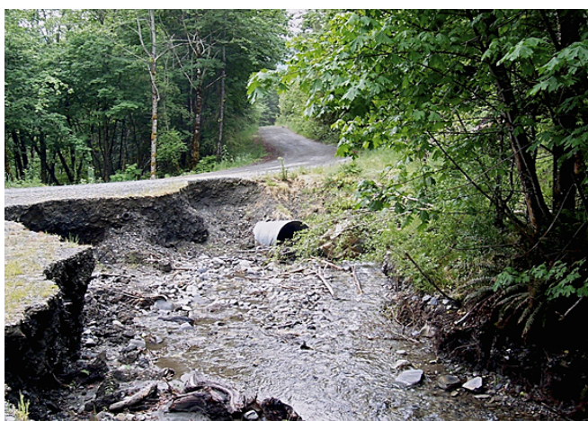
Figure 18. This culvert plugged with debris during a storm. Although it is still in place, the swirling water and debris caused extensive erosion of the road and the adjacent old log landing. This type of failure is common on older “legacy” roads where crossings were not adequately designed to pass 100-year flows plus debris and sediment. In many cases, the culvert will be displaced and transported downstream.
