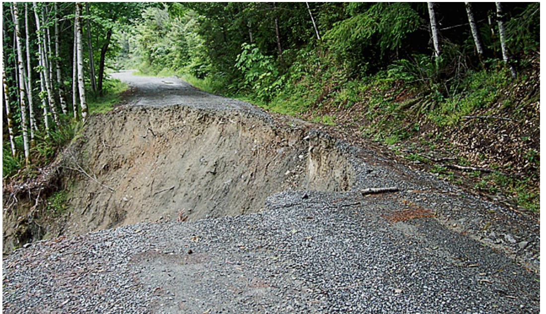
Figure 3. Stream undercutting at the base of the slope below the road caused this landslide. Photo: Richard Harris.
