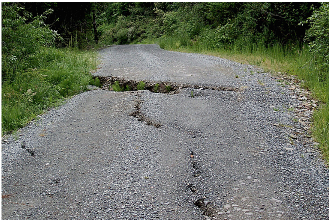
Figure 21. Cracks appearing in the road surface, especially at the edges of fills, are a sure sign of an impending failure or landslide. The horsetail growing in these cracks indicates that the source of the problem is groundwater seeping through the road bed. Photo: Richard Harris.
