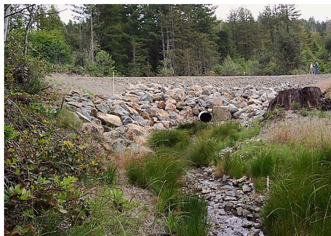
Figure 19. This reconstructed stream crossing on an all-season road used for hauling timber illustrates many desired design features. The culvert is sized to accommodate 100-year storm flows plus debris and sediment. It is located at the base of the road fill at the elevation of the channel to prevent scour. The face of the crossing fill is armored with rock. The road has a critical dip to prevent diversion and is surfaced with gravel.
