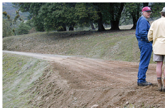
Figure 11. This rolling dip has a gentle increase in grade going left to right and a reverse grade (where people are standing) to direct water off the road at the dip. Photo: Gary Nakamura.
