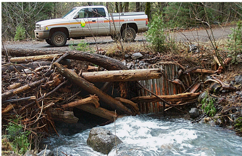
Figure 20. This extreme case of culvert blockage at a stream crossing was caused by a large storm event. All culverts should be inspected before and after storms to ensure that they are clear. Photo: © Angela Wilson; used with permission.
