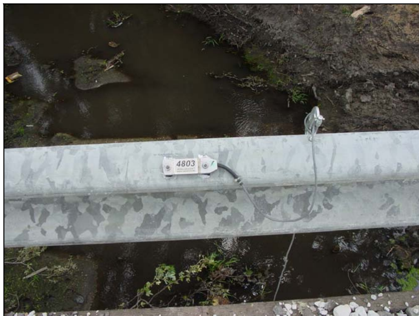
b. Strain transducer on guard rail.
