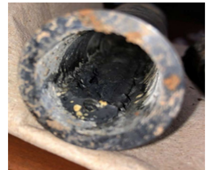
Figure 1: Degraded plastic pipe post-wildfire. PC: CA State Water Board Division of Drinking Water
