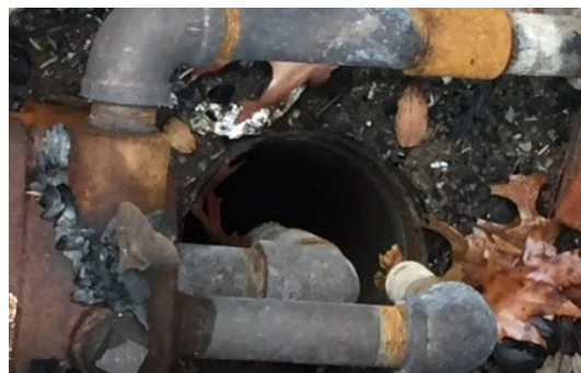
Figure 4: Charred well pump and piping. PC: Tennessee Department of Health
