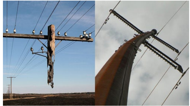
Figure 4: Various types of ways utility poles can be damaged by fire. Photo: Woodpoles.org
