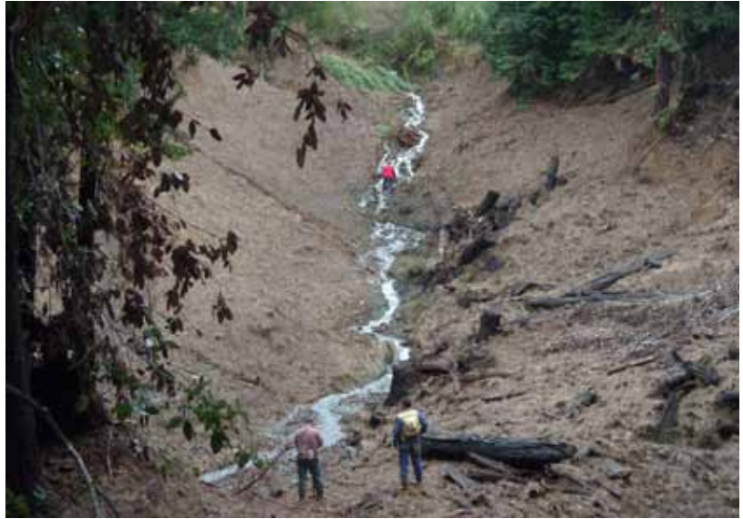
The Little Pepperwood Creek Planning Watershed landing filled in the headwaters of the creek. It was removed and the headwaters brought back down to their natural grade. 13,000 cubic yards of sediment (that’s 1,300 dump truck loads!) were removed from the site. That sediment would have eventually eroded into the stream network.
