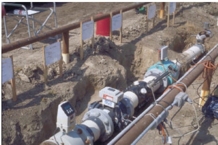
Danfoss, ISCO, Marsh McBirney, and Water Specialties meters at flow meter test in Tulare County
