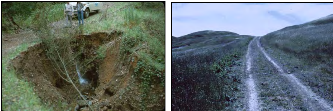
Figure 21: Examples of ranch road maintenance implemented in Lagunitas Creek Watershed following the 1982 flood in cooperation with Marin County Fire Department showing extensive erosion around a culvert outlet (left), and an upgraded road with out-sloped grade and water bar (right).
