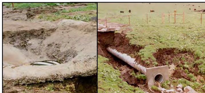
Sediment plugged inlet caused failure of Water Control Structure.
