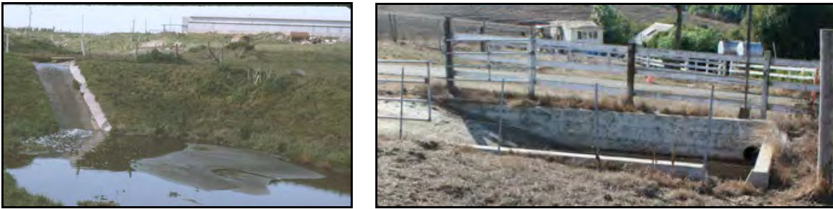
Figure 29: Examples of Sediment Basins depicting a large-scale design constructed in the 1980s (left), and a smaller version with a paved access ramp to facilitate maintenance built in 2005 (right).
