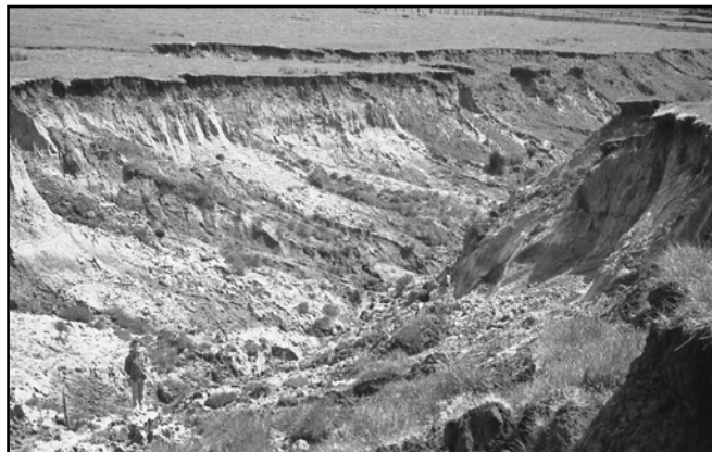
Stopping gully erosion like this was a motivation for forming the Marin RCD.
