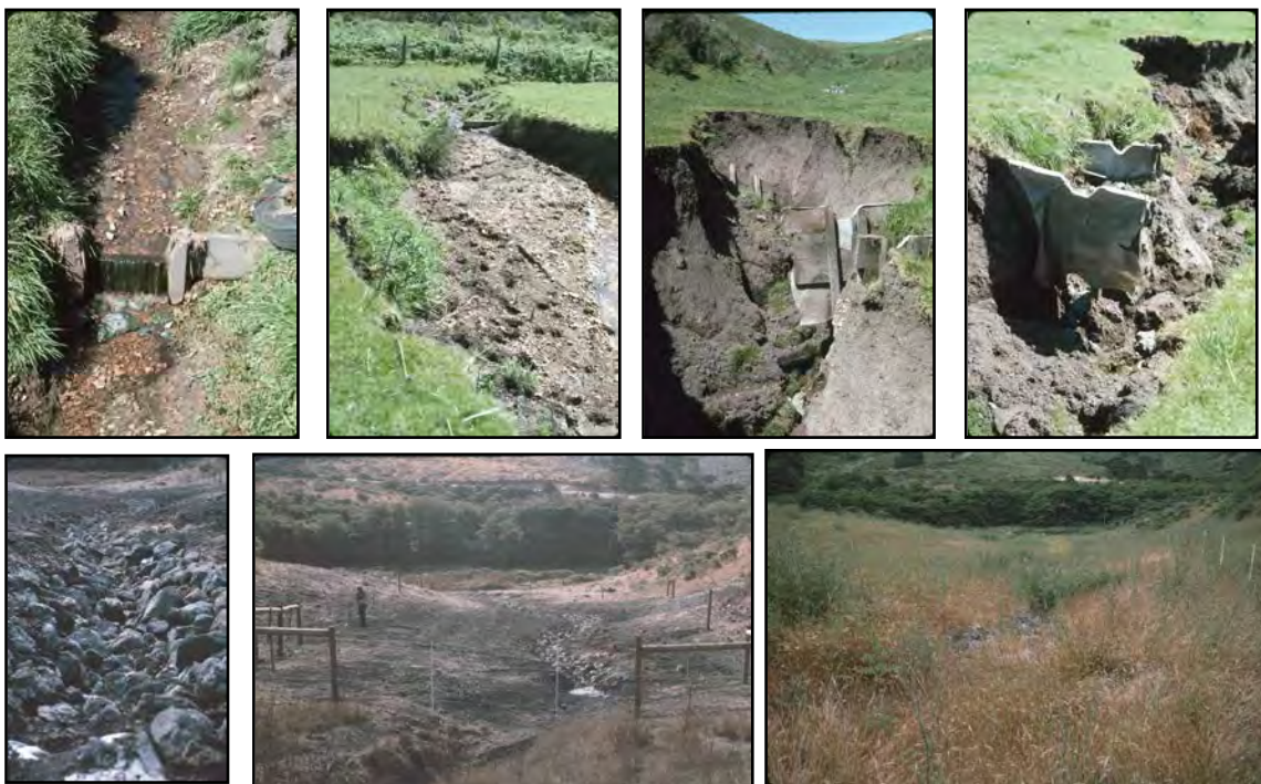
Figure 32: Photo monitoring of a grade stabilization project with functional redwood board checkdams before March 1986 storms (top left 2 photos), following March 1986 storms (top right 2 photos), the emergency repair installed a Lined Waterway with control fencing (bottom left 2 photos), and one year later in June 1987 (bottom right). Designed by NRCS.
