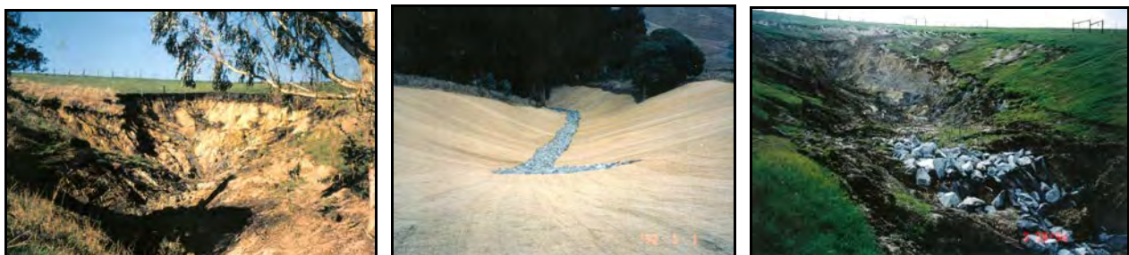
Figure 34: An eroding gully pre-project (left), after implementation of Lined Waterway and other practices in 1992 (middle), and four years later the site had unraveled (right).
