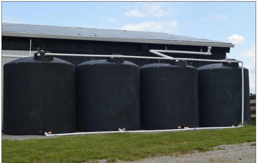
Figure 4. Harvesting water from a roof can provide producers with an alternative water source that is both clean and inexpensive. Photo by Lee Moser
