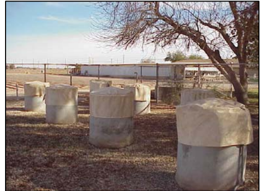
Desert REC Treated Water Storage Cisterns
